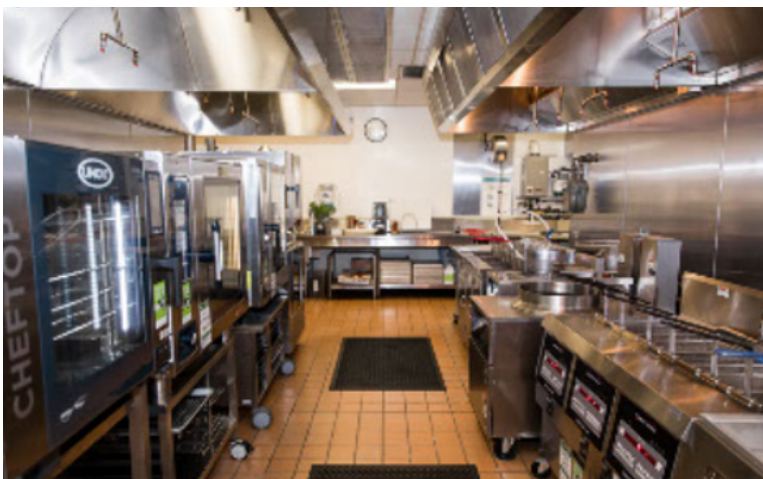
Commercially approved, installed and operational kitchen ventilation with commercial gas equipment properly installed beneath.
